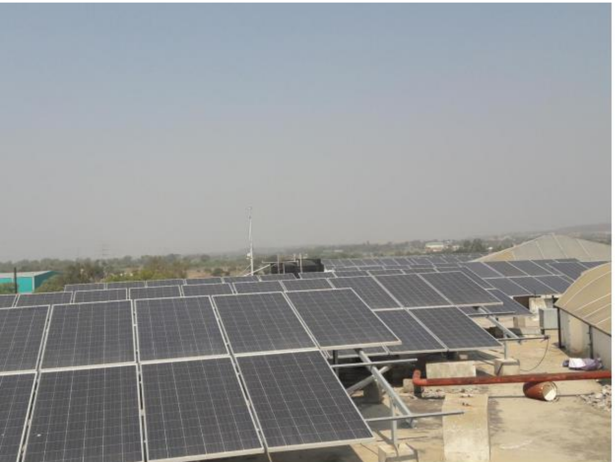
Rooftop Solar Power Plant
