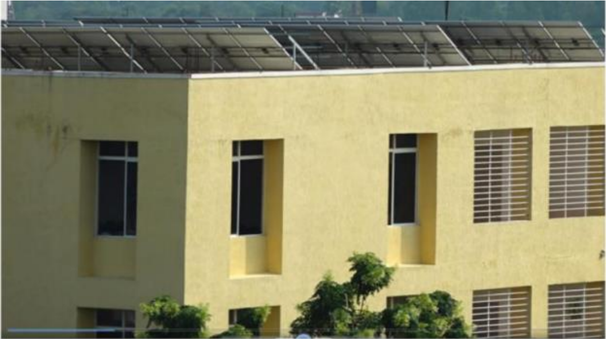
Rooftop Solar Power Plant
